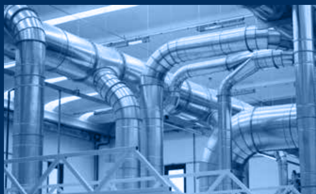
vista impianto interno /internal plant view
