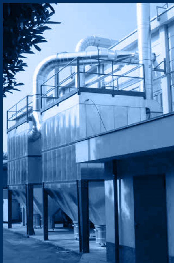
vista filtro a maniche / sleeve filter view
