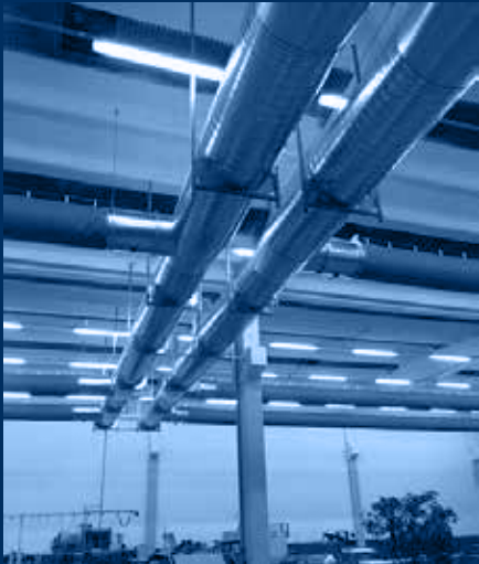
vista distribuzioni interne al reparto / internal view of air distributions with jet-in duct
