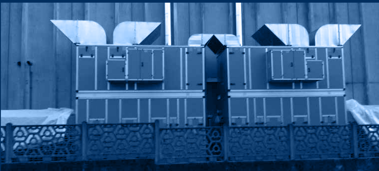
vista globale esterna impianto /external global view of the plant
