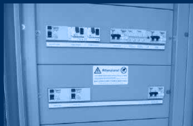
vista quadro centrale elettronica /electronic control cabinet view
