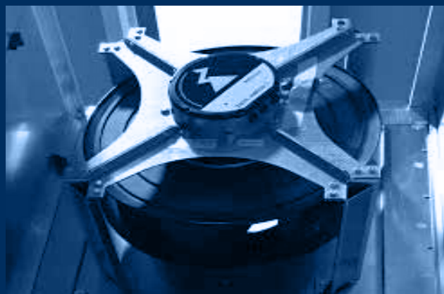
vista interna UTA - sezione ventilatori plug fan / internal view of air handling unit - plug fan
