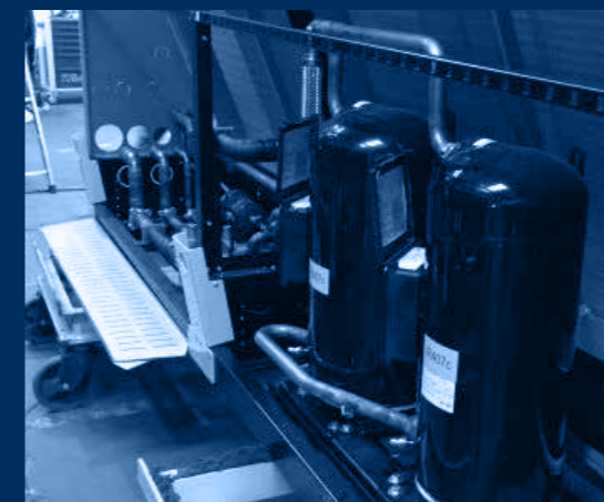
vista circuito frigorifero / refrigerant circuit view
