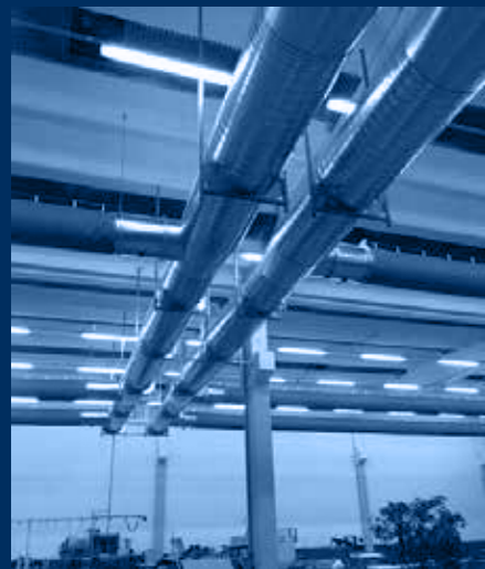
vista distribuzioni interne al reparto / internal view of air distributions with jet-in duct
