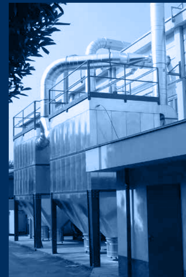
vista filtro a maniche / sleeve filter view
