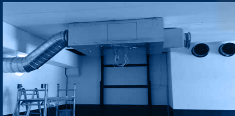
vista UTA e circuiti aeraulici /AHU and aeraulic circuits view
