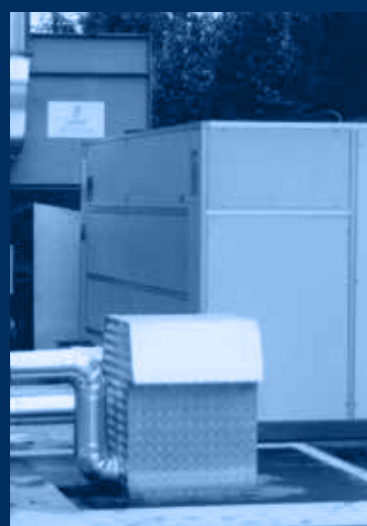
vista refrigeratore e box pompe / cooler and box pumps view
