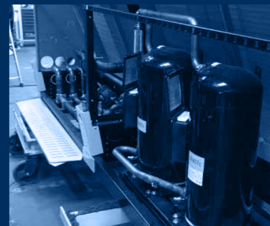
vista circuito frigorifero / refrigerant circuit view
