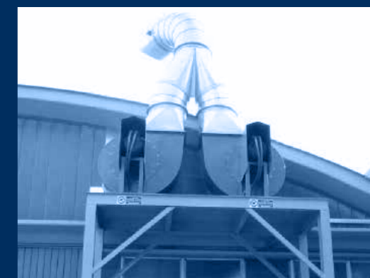
vista impianto esterno /external plant view
