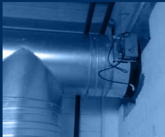
vista serranda tagliafuoco in attraversamento reparto / fire damper view in wall crossing between departments
