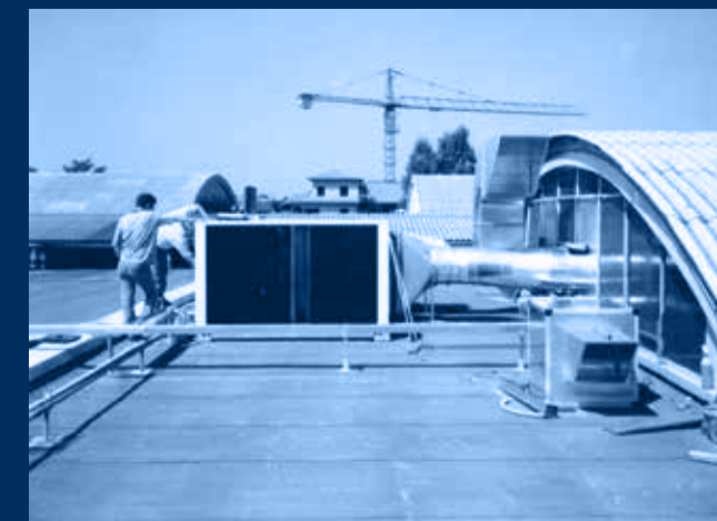
vista macchina in copertura / plant's view on the roof
