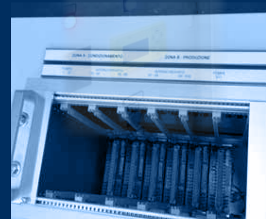
vista rack schede rilevatori gas / gas detectors rack view
