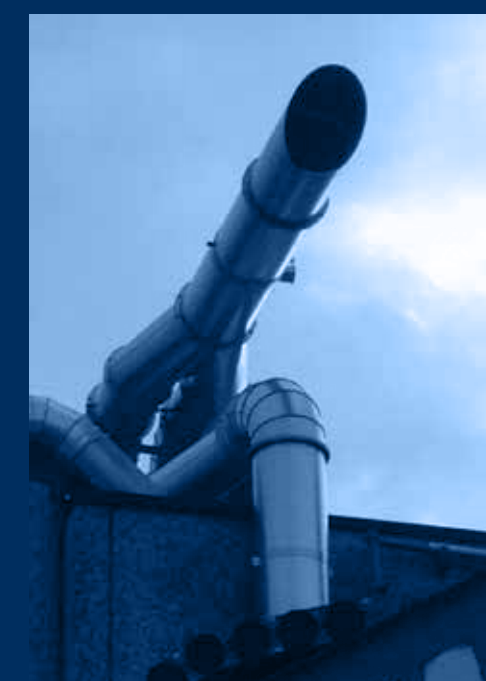
vista espulsione aria / exhaust air view
