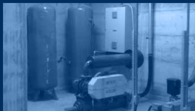
vista interna Centrale vuoto spinto/internal view of pushed vacuum station
