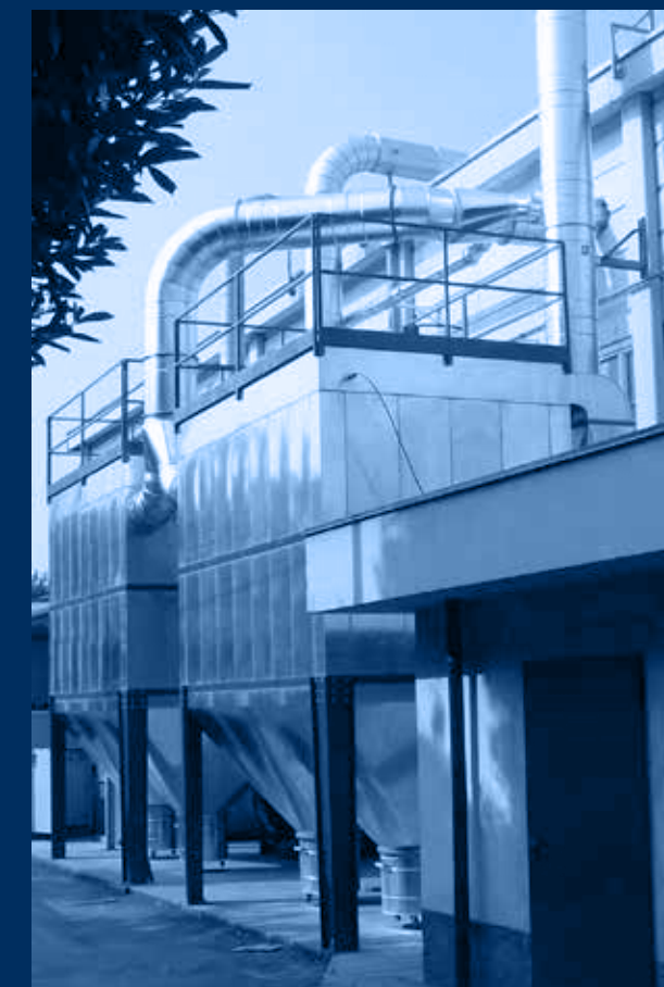
vista filtro a maniche / sleeve filter view
