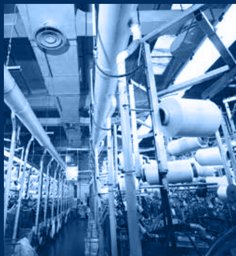
interno tessitura / inside of weaving department
