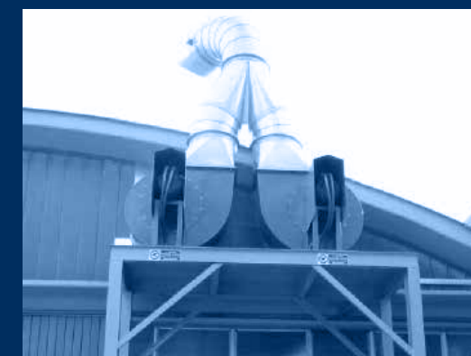
vista impianto esterno /external plant view
