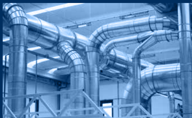
vista impianto interno /internal plant view
