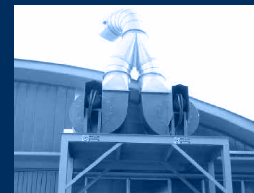
vista impianto esterno /external plant view
