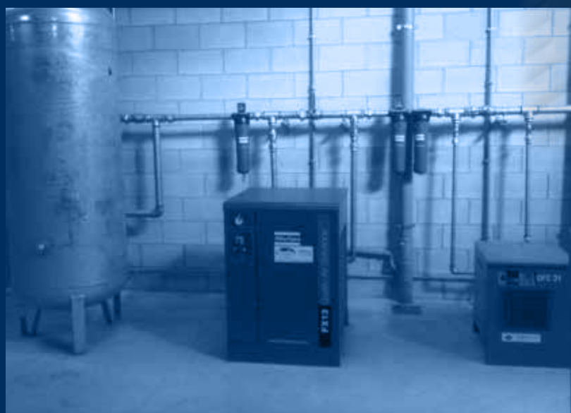
vista interna Centrale aria compressa /internal view of compressed air station
