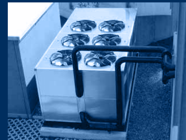
vista refrigeratore/cooler view
