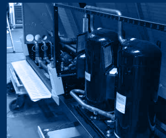
vista circuito frigorifero / refrigerant circuit view
