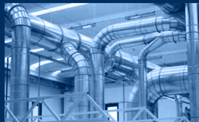
vista impianto interno /internal plant view
