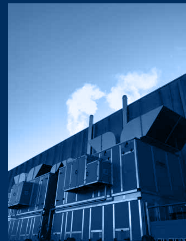
vista globale impianto esterno / external global view of the plant
