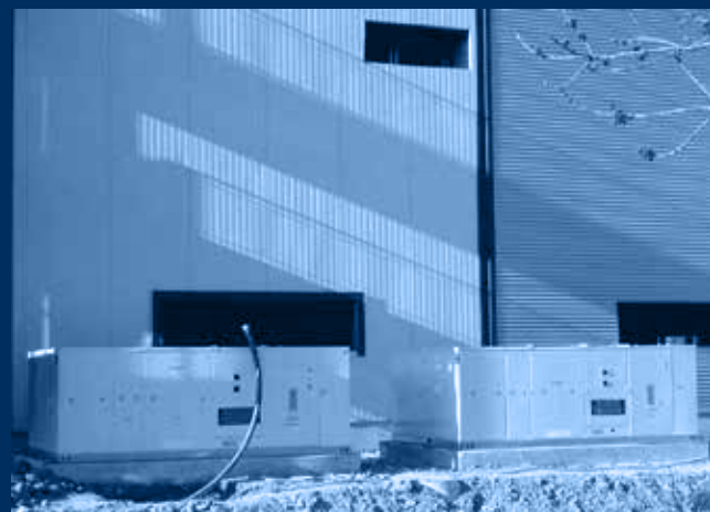
vista macchine esterne / external machines view
