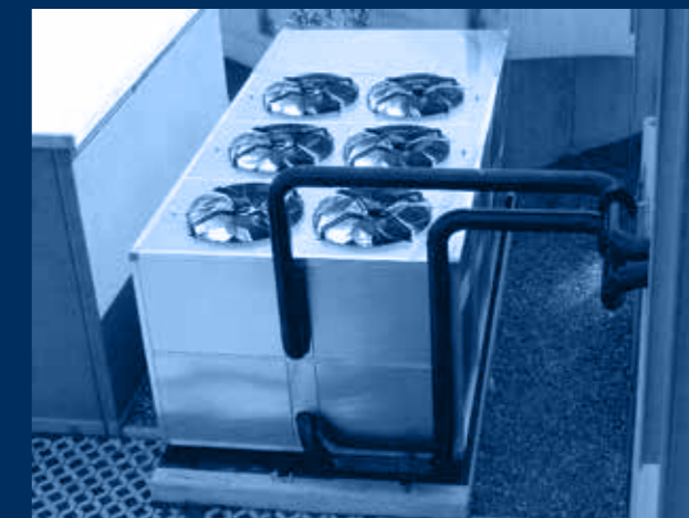
vista refrigeratore/cooler view
