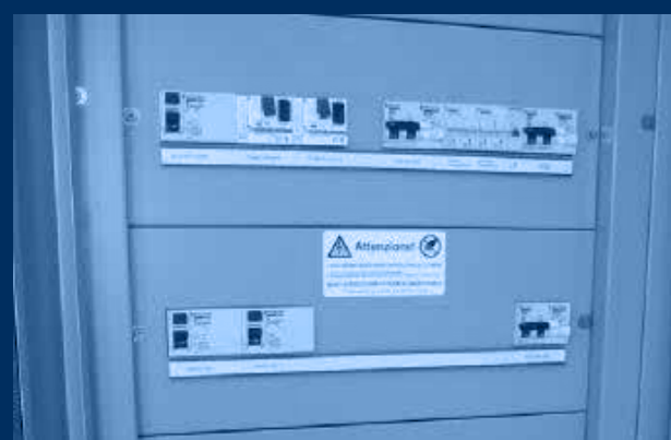
vista quadro centrale elettronica /electronic control cabinet view
