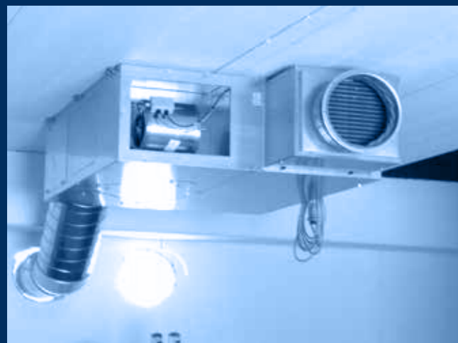
vista UTA sala Commiato /AHU's view of Funeral home
