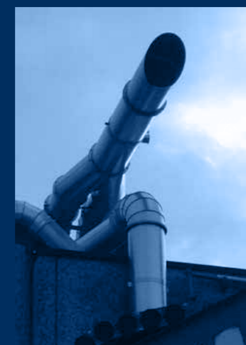
vista espulsione aria / exhaust air view
