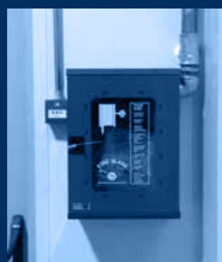
vista idranti interni UNI 45 / internal hydrants UNI 45 view
