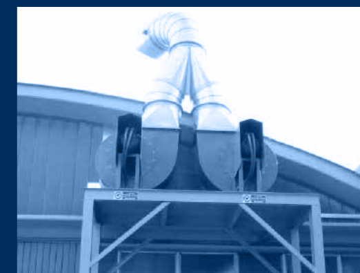
vista impianto esterno /external plant view
