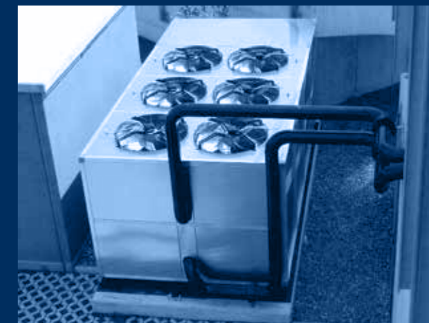
vista refrigeratore/cooler view
