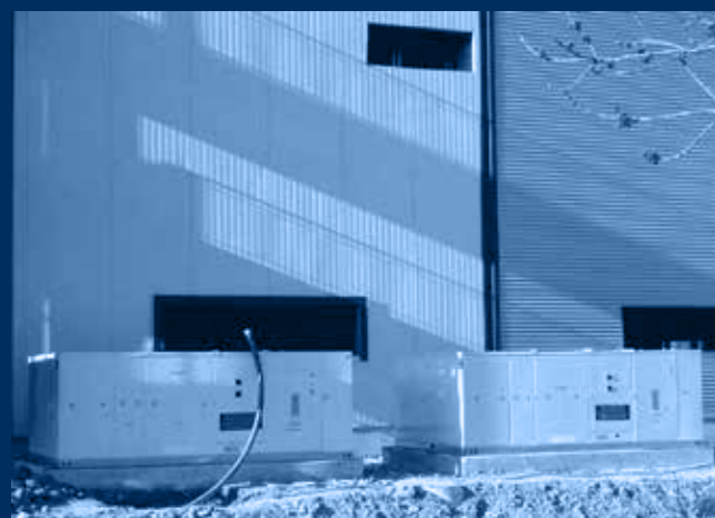
vista macchine esterne / external machines view
