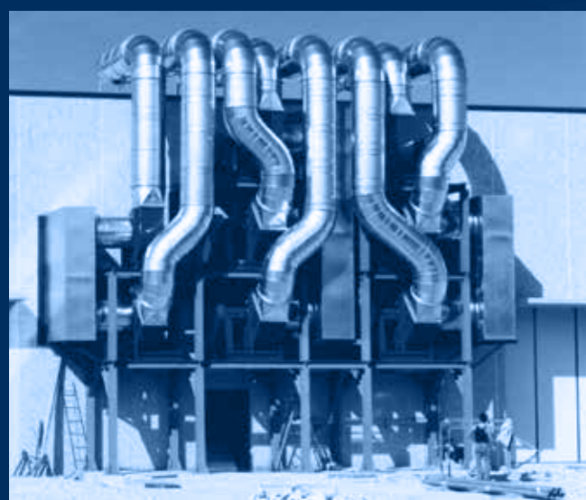
vista impianto esterno completato / external completed plant view
