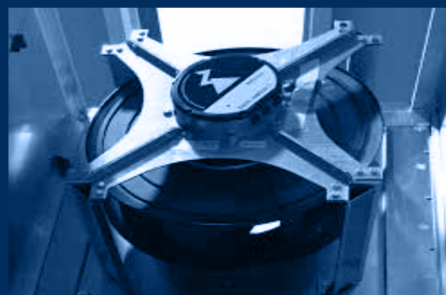
vista interna UTA - sezione ventilatori plug fan / internal view of air handling unit - plug fan
