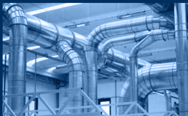
vista impianto interno /internal plant view
