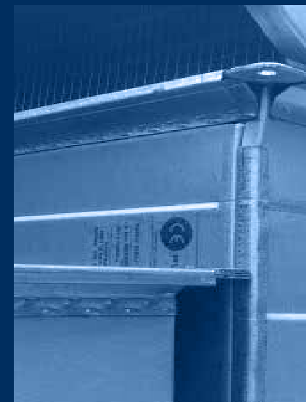
vista condotte certificate CE per impianto SEFFC /certified CE ducts view
