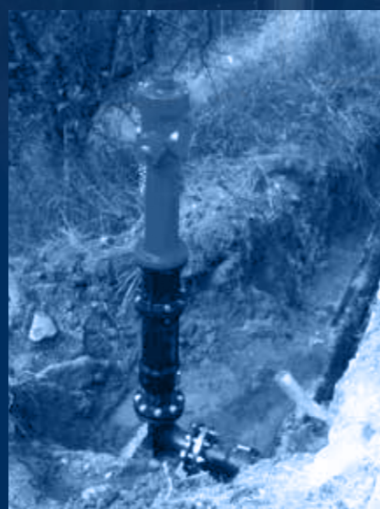
vista idranti esterni UNI 70 /external hydrants UNI 45 view
