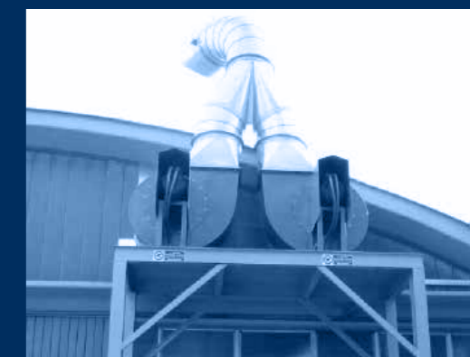
vista impianto esterno /external plant view
