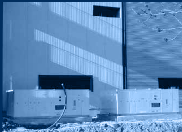
vista macchine esterne / external machines view
