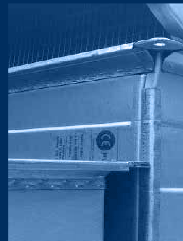
vista condotte certificate CE per impianto SEFFC / certified CE ducts view
