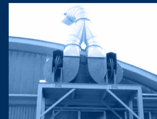
vista impianto esterno /external plant view
