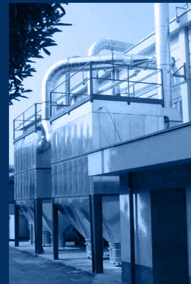
vista filtro a maniche / sleeve filter view
