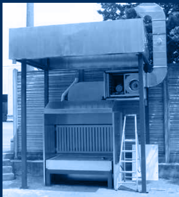
vista cabina aspirante completa /complete suction cabin view
