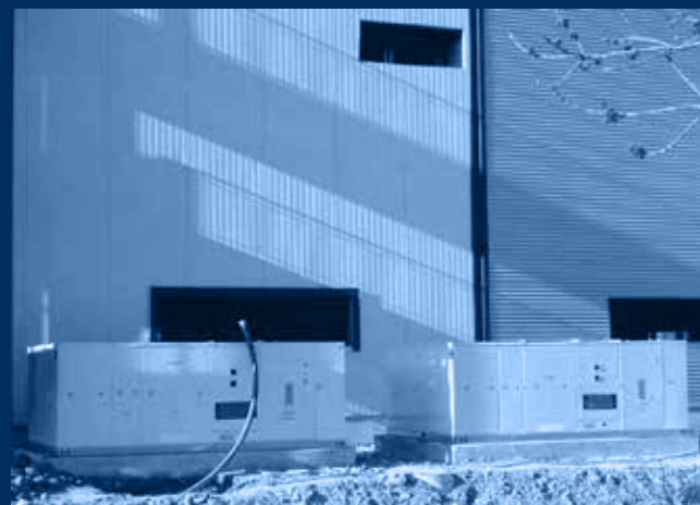
vista macchine esterne / external machines view
