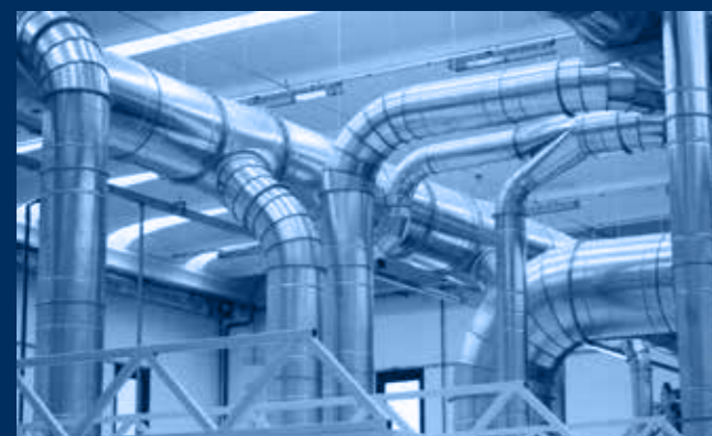
vista impianto interno /internal plant view
